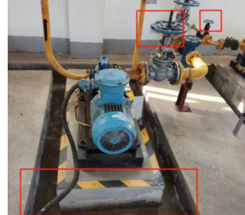
泵房内手动阀、逆止阀、导流槽
